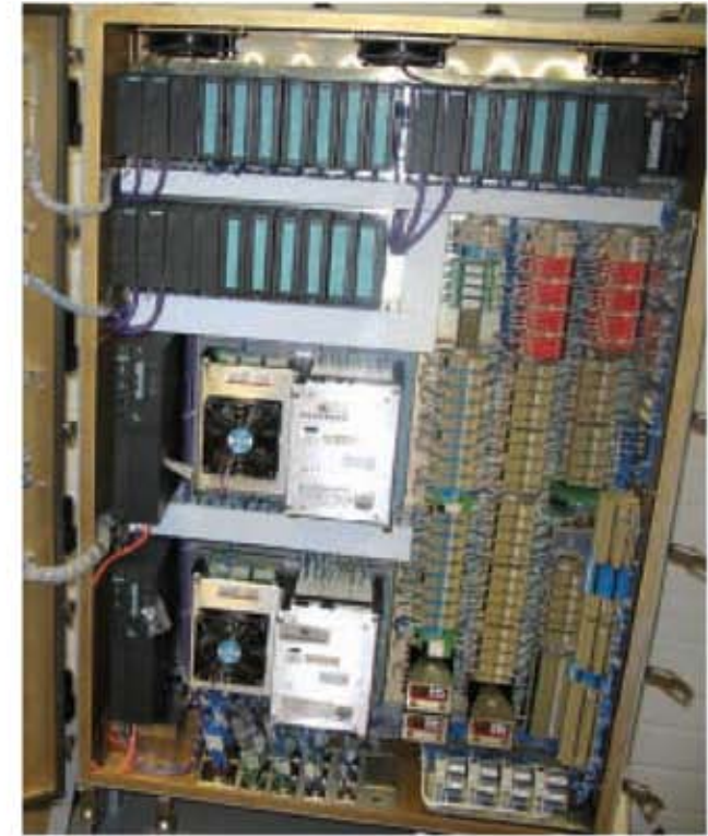
Gas turbine controls.
